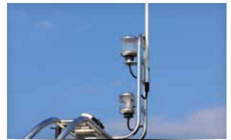
Zero loss – no degradation of radio performance
